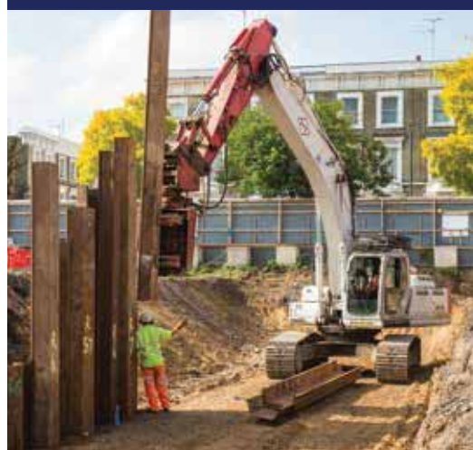
The first concrete beams are cast around the perimeter of the site at Lillie Square
