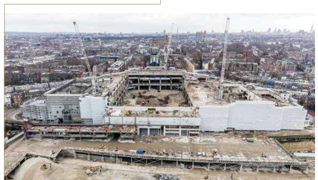
EC2 roof and structures demolished and the roof of EC1 demolished and removed from site
