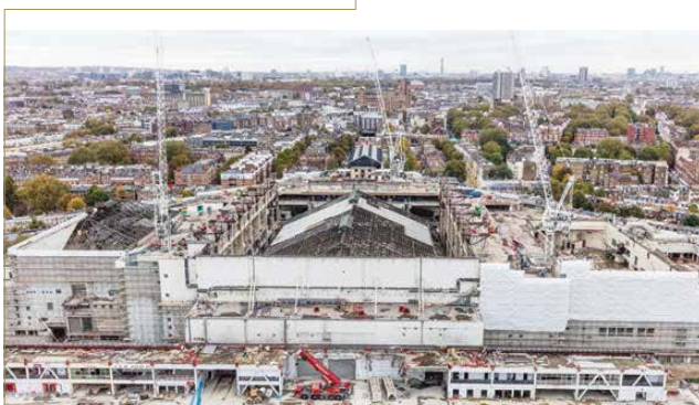
The 1,300 tonne roof of EC1 was lowered in an eleven-hour, precise operation
