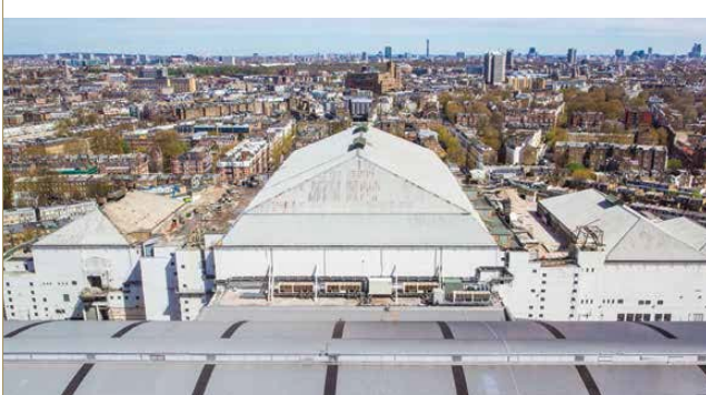
The services within EC1 and EC2 were decommissioned in early 2015 as internal deconstruction of the buildings began
