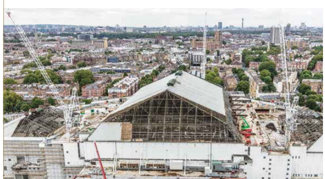
By summer 2015, all internal demolition complete and roof trusses prepared for demolition
