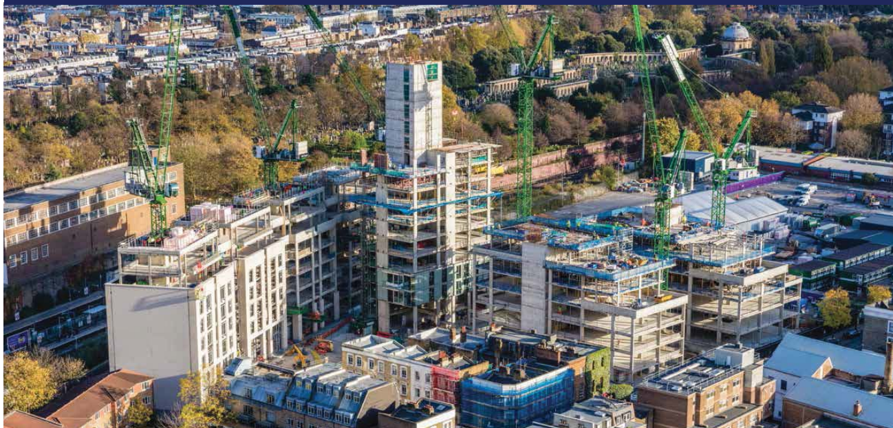
Construction progress on site at Lillie Square. The first Phase 1 buyers are to begin moving in during 2016
