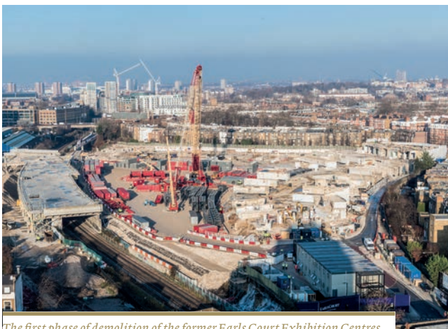
The first phase of demolition of the former Earls Court Exhibition Centres completed in 2016. The Heavy Lifting Crane was introduced for enabling works to prepare the site for further use
